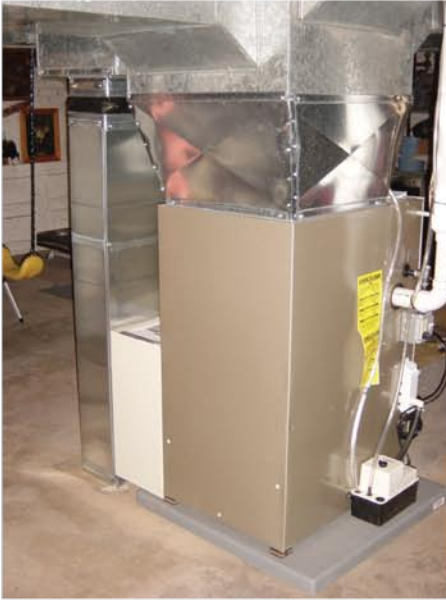
The Fishers' new Carrier Infinity furnace with Aprilaire media filter and humidifier, and Little Giant condensate pump.
