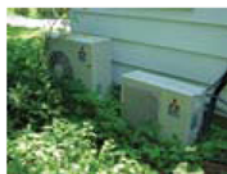
The outside compressors for downstairs and half the upstairs.
