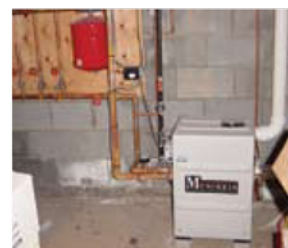
The boiler and manifold.
