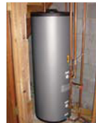
The domestic hot water tank.
