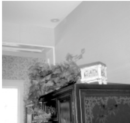
The Unico air conditioning outlet looks like recessed lighting in the ceiling.
