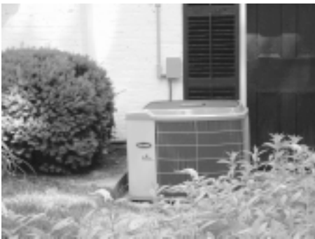
The Carrier WeatherMaster compressor for the main air conditioning system.
