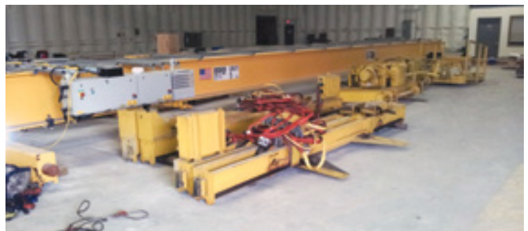
Overhead crane to be installed
