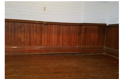
Floor settlement at corner
